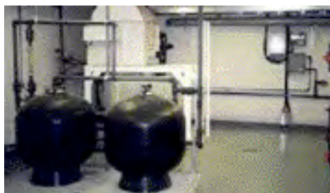
Process room showing sand filters at Mill Bay
